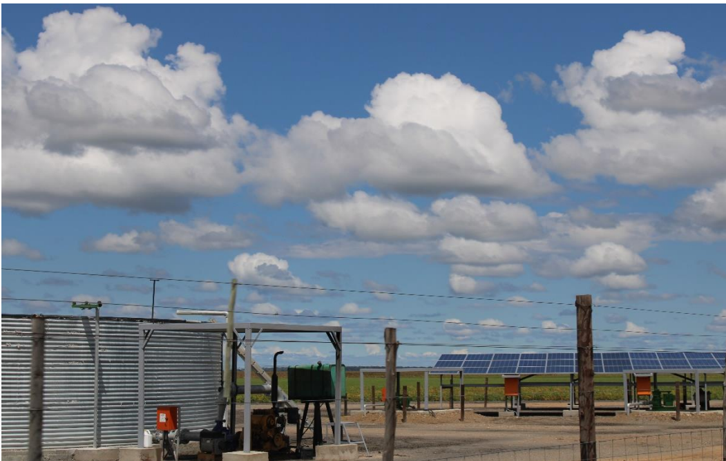
Plate 1: Solar powered boreholes and water reservoir installed at one of the farms
